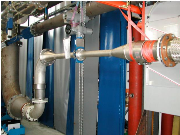
VACOMASS® calibration of the measuring and control section
